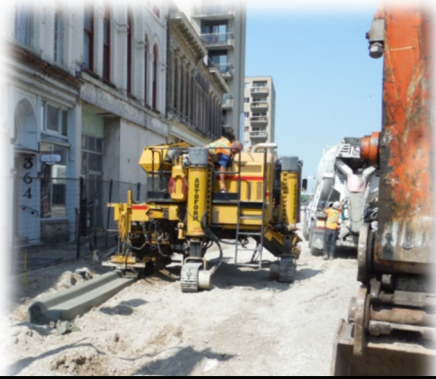
Example of curb machine placing curb in last Phase of Talbot Construction
